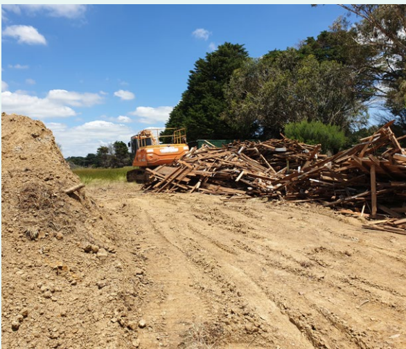
Photo: Illegal dumping of demolition waste, including asbestos, in Whittlesea.
